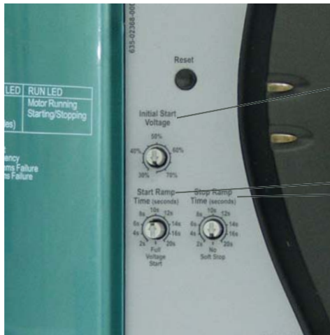
CSX control panel
